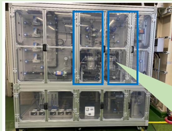
吸着塔A 吸着塔B
